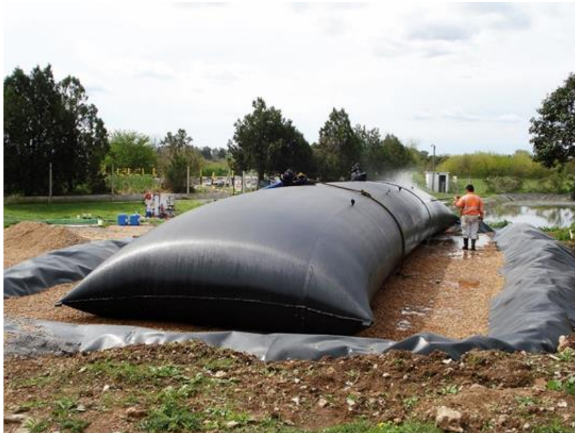
Geotextile tubes used for capturing and further dewatering sludge for disposal in solid form
