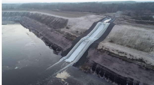
Inlet with a maximum inclination of 1:1,5 and an approx. length of 160 m for a max. discharge of 5 \text{ m}^3/\text{s}
