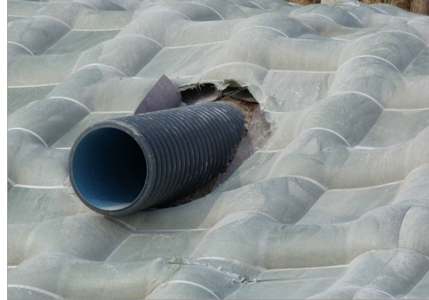
Close up: mouthing drainage pipe
