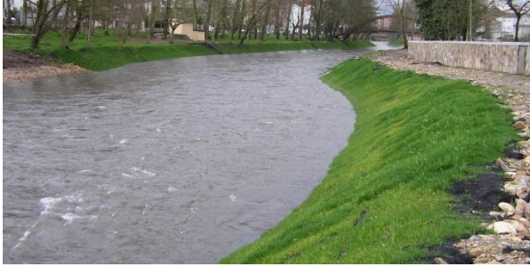
b. Heavy geomat filled with crushed stone/bitumen and vegetation growing through the mat
