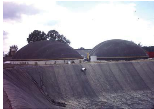
Anaerobic digesters with waste lagoon
