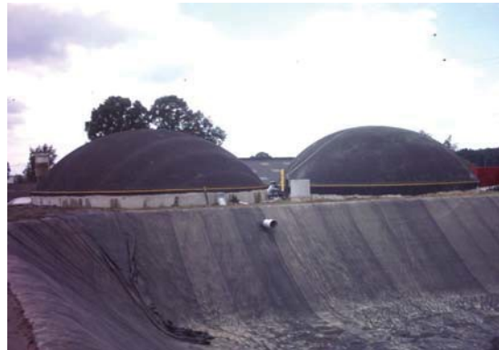
Anaerobic digesters with waste lagoon
