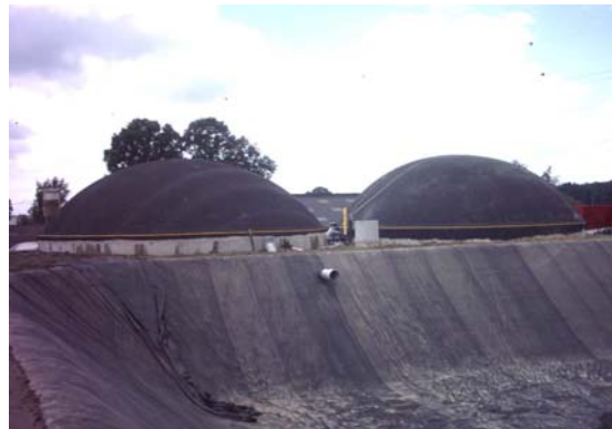
Anaerobic digesters with waste lagoon
